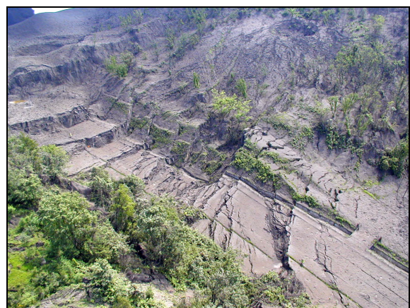
Old National Road 230 Graben, taken from northeast side on July 2, 2000 Courtesy of C. Inaba
